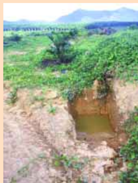
> During periods of heavy rainfall silt pits and roadside soakaways retain water and soil run-off
